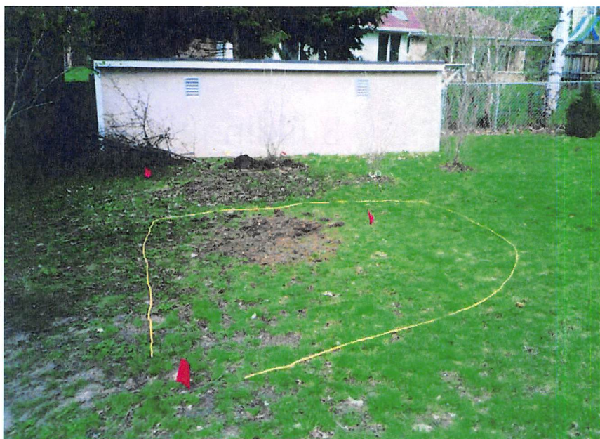
The perimeter of a rain garden is defined with string before digging.
